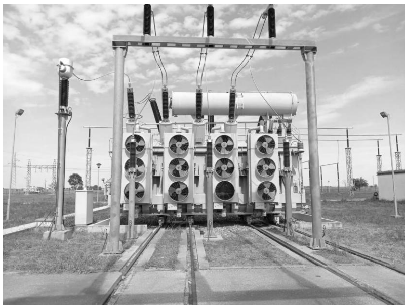
Slika 6. Transformator Shenbian 400 /110/10 kV/kV/ kV, 300MVA
